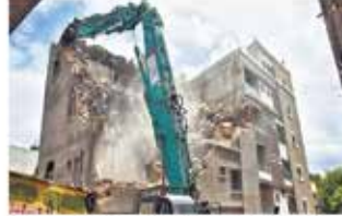
A large excavator is demolishing a multi-story building that is leaning significantly. Debris is visible at the base of the structure.
