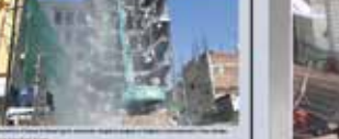
A demolition site with a large excavator and a partially destroyed building structure.
