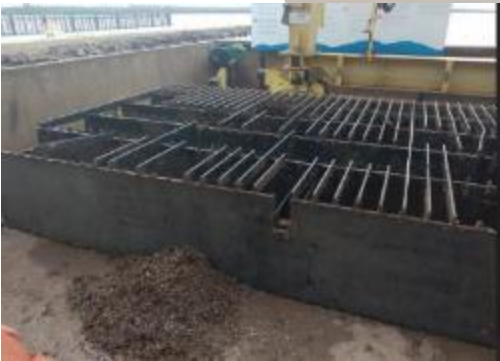
Damaged intake trash rack
